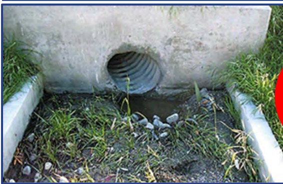
Pipe Condition BEFORE Damage (as-designed pipe condition)
