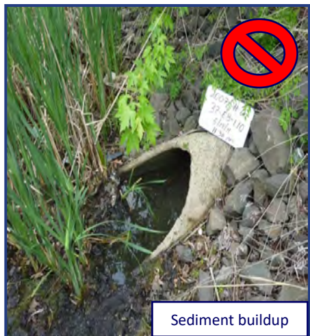
Eroded emergency overflow
