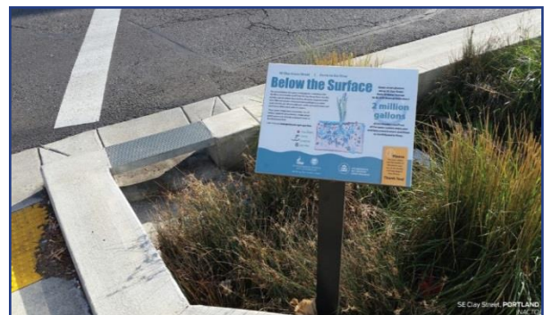
Figure 3-22. Signs to Assist Maintenance Staff
