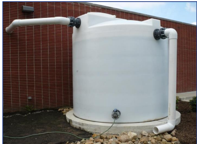
Photo: Cistern used to capture runoff from the rooftop and irrigate a nearby bioretention BMP. (Source: Wood E&IS)
