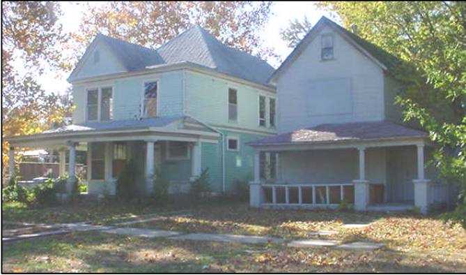
Two large vacant and deteriorating homes along the west side of Clay Street (Tennessee Town neighborhood).
