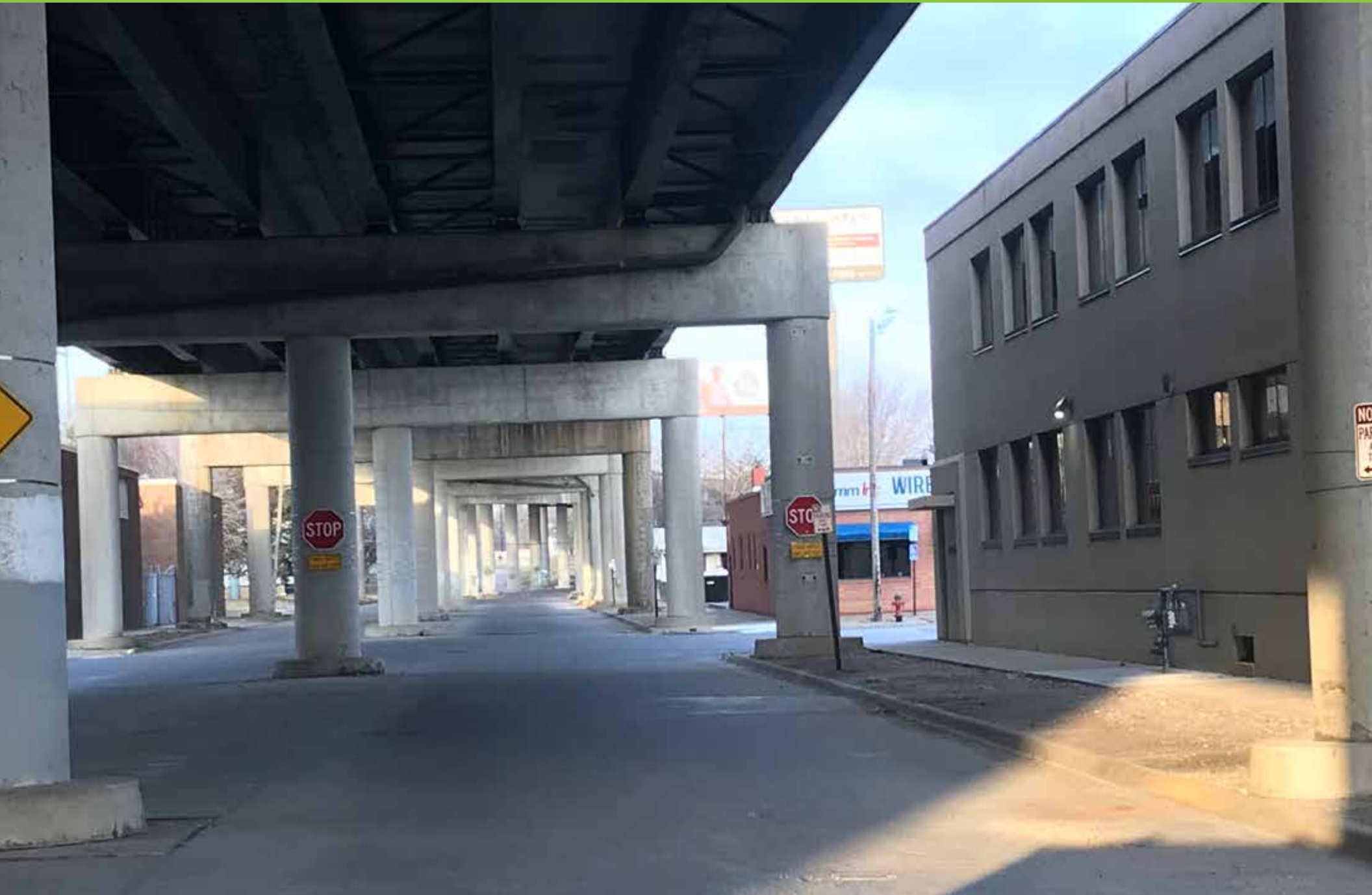
The Polk-Quincy viaduct is the primary gateway into River South. Proposed improvements should include public art to reflect the authenticity of the neighborhood. Image courtesy of Stantec
