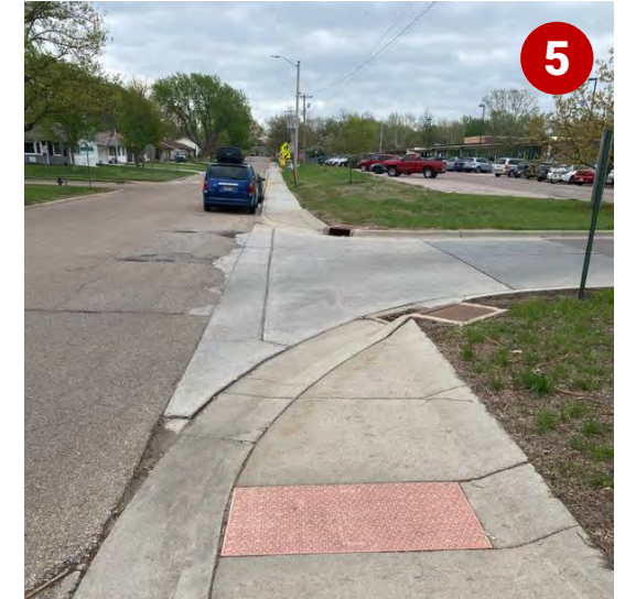
Missing crosswalk marking and ADA compliant curb ramp near school on SW 29 th Terrace
