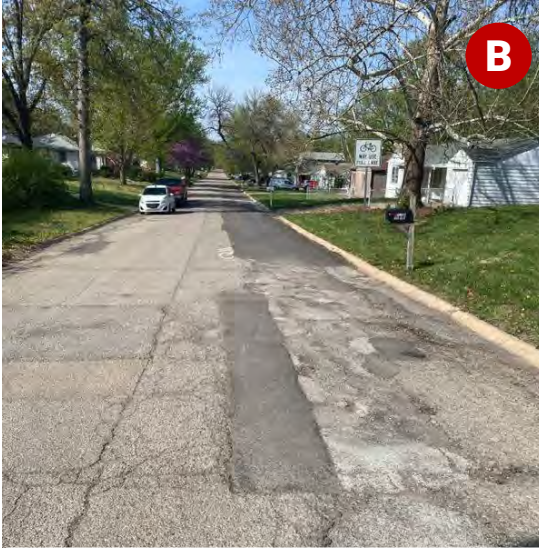
Existing sharrow covered with asphalt (SE Wisconsin Ave)
