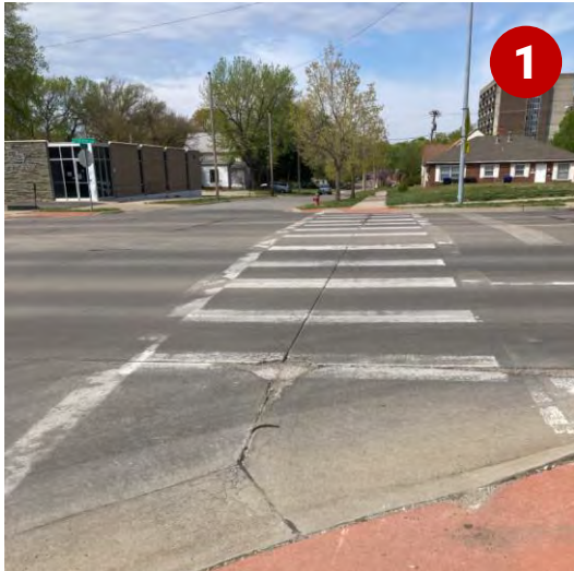
Faded crosswalk markings, lack of detectible warning surface at SW Topeka Boulevard and SW 14 th Street
