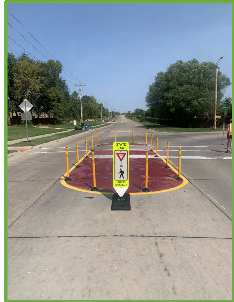
Pedestrian Safety Island demonstration project on Green Valley Road in Manhattan, KS
