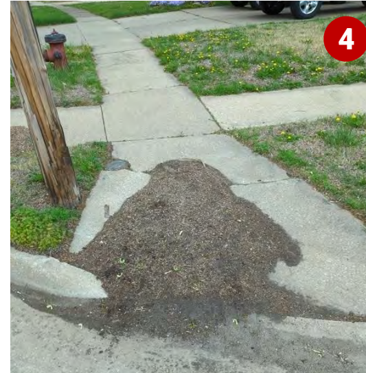
Missing ADA compliant curb ramp and obstructed at SW Burnett Road and SW 30 th Street intersection
