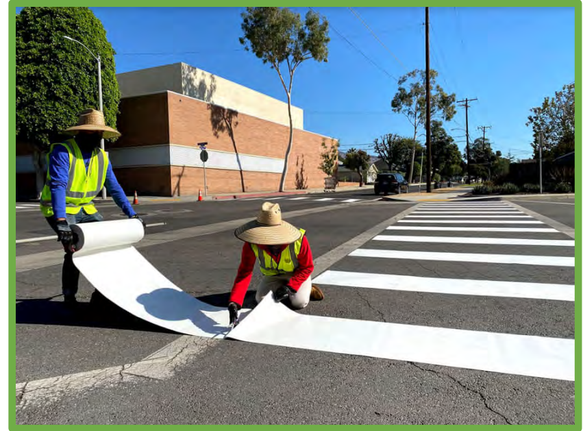
1Active SGV Staff install a crosswalk demonstration project in the San Gabriel Valley in California
