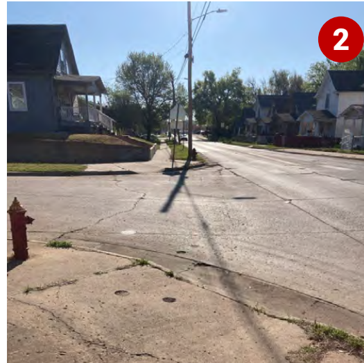
Lacks ADA compliant curb ramps, and missing crosswalk markings and signage at SE 17 th Street and SE Quincy Street
