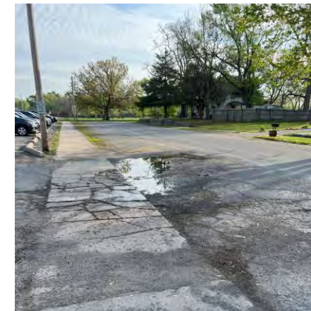
Poor pavement conditions on NE Monroe Street
