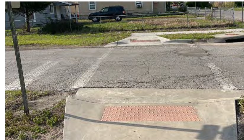
Faded crosswalk markings faded at SE 5 th Street and SE Lamar Street intersection
