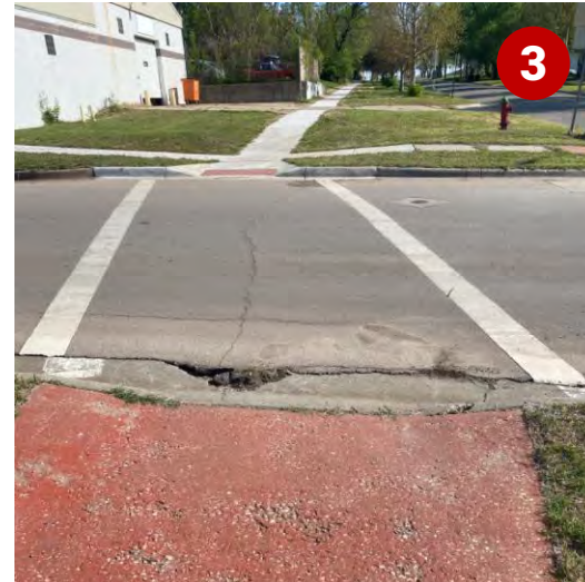
Ramps lack detectible warning surface and crosswalk markings faded at SW 13 th Street and SW Monroe Street
