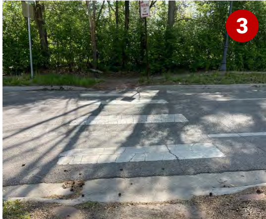
Faded crosswalk marking and missing ADA compliant curb ramp (SW Munson Ave and SW Washburn Ave)
