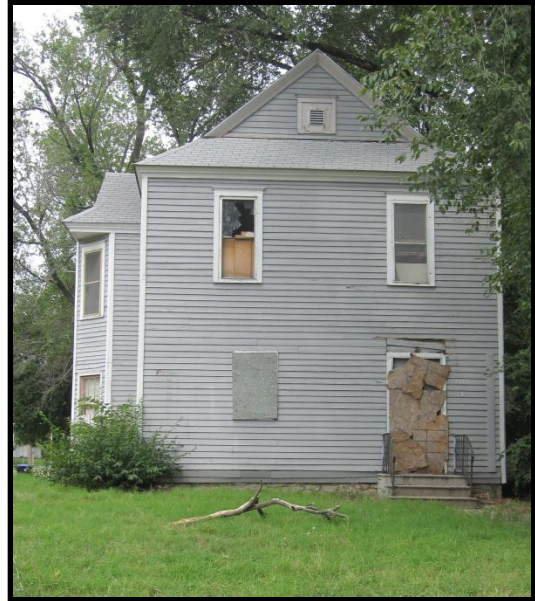
Abandoned house (1503 NE Quincy) directly across from the Quincy Elementary School main entrance
