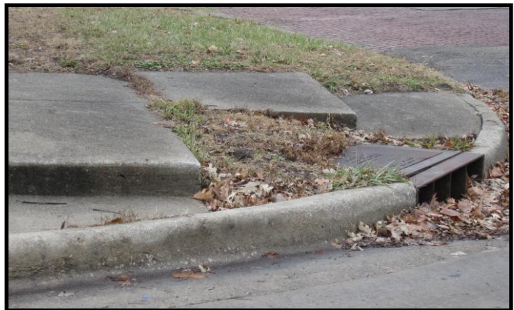
Lack of access ramps at SE corner of NW Jackson St. and NW Grant St. with overgrown sidewalks
