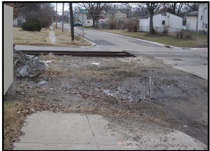
End of sidewalk before railroad crossing at NW Tyler St. and NW Morse St. forcing pedestrians to cross in the street
