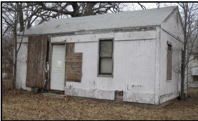
An abandoned house (807 NW Gordon St.) where stray dogs were coming in and out of the structure
