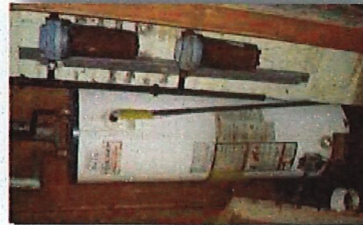
Hot Water Heater Placement
